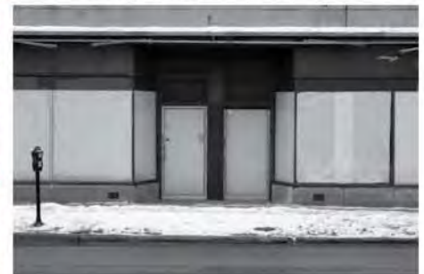
One of many vacant buildings along Milwaukee Avenue
